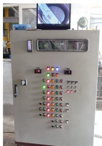
Fig 5. Column Control Panel
