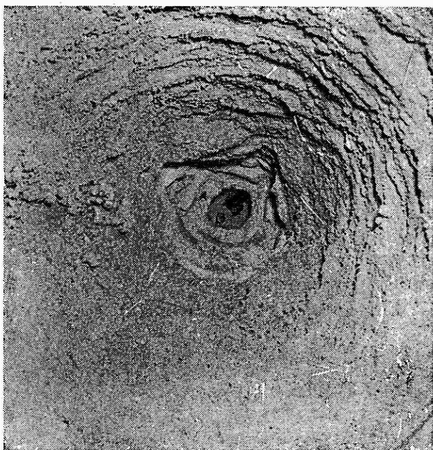
Fig. 1 The Kiln build up as seen from the discharge end. At 'A' the internal diameter is 11 inches and at 'B' it is only 7 inches.
