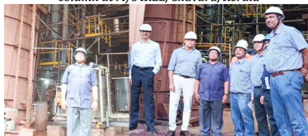
Figure 9: Commissioning of a pilot plant at the Premises of at M/s JSW Steel, Toranagallu, Karnataka.: CSIR-NML designed an entire system for processing low-grade iron ore using column flotation.
