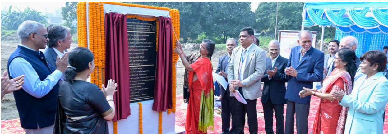
Figure 3: Foundation stone laying by DG, CSIR in the presence of NML-Research Council members, Director CSIR-NML, Former Directors, CSIR-NML and other dignitaries on November 26 th , 2024 at Magnesium Plant Area
