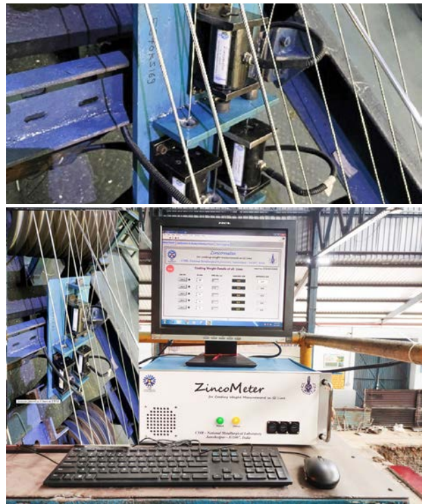
Figure 10: Zincometer system with 3 sensors installed in the pad wiping line at Tarapur Wire Mill (TWM) of Tata Steel
