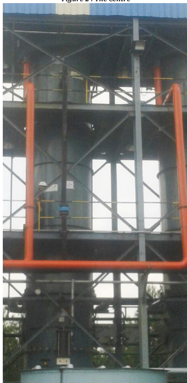
Figure 3 : Commercial scale flotation columns for barite (1000 tpd) at M/s Oren Hydrocarbons (P) Ltd., Chennai
